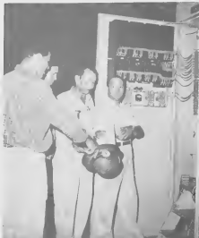
ELECTRICIANS AND instrumentmen were involved in the testing and switching. Facing the camera, above, are Sylvester Geerman, Powerhouse No. 1 electrical foreman, and Max Emmannuels, tester. The center shows four of the group comparing notes on the progress of the tests which preceded the tying in of the government's electrical power to the refinery's electrical system. In the center of the group is J. J. Lavell of the Public Utilities Department of the Aruba Government. He is flanked by C. F. J. Peeren of Mechanical-Electrical, H. F. Gaba of the Technical Department and C. R. Osborn of Process-Utilities. Three of the group, right, test out facilities in the government's substation at the former cold storage site. Mr. Lavell is closing a breaker. Prior to this, a fault was simulated to assure the technicians that the breaker was functioning correctly.
